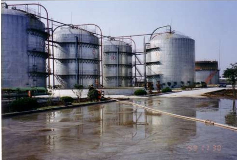
Tank group for anaerobic fermentation
