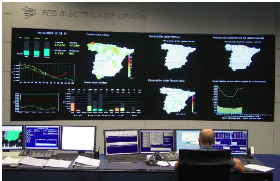
Fig 3-12 The control center of REE
