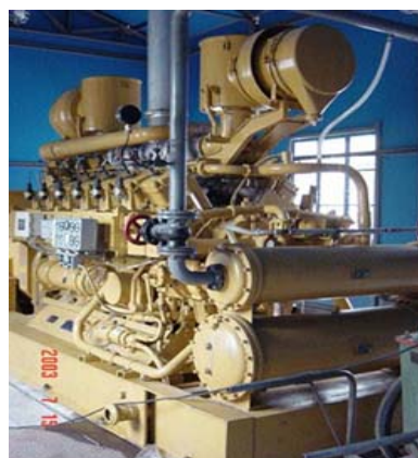
Fig.5-5 highly effective anaerobic biogas power generation unit
